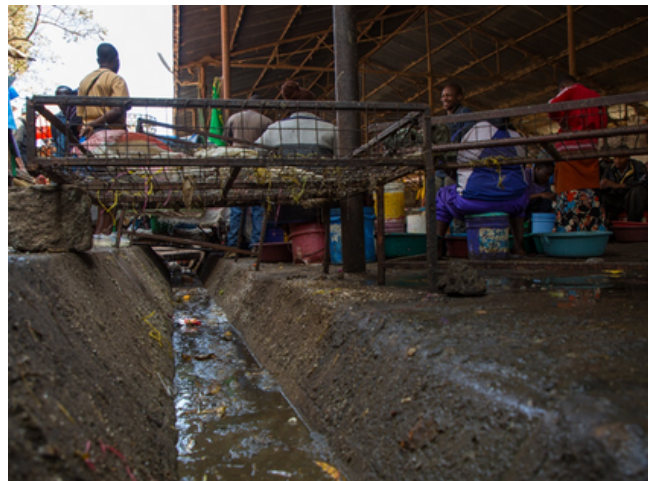
DRAINAGE SYSTEM AT KILOMBERO
